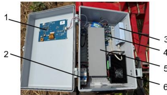
Fig. 2 - Control Cabinet Hardware Structure 1-TJC1060X570 display screen; 2-Terminal block switch; 3-5V power supply; 4-STM32F411RCT6 microcontroller; 5-Cable tray; 6-MSSD-60LMA motor driver
