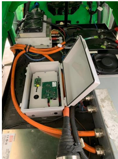
Fig. 3 - Physical placing of the router in the tractor
