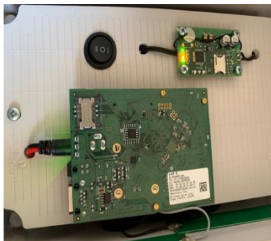
Fig. 2 – Mounting of the Access Point and the remote control board in the box
