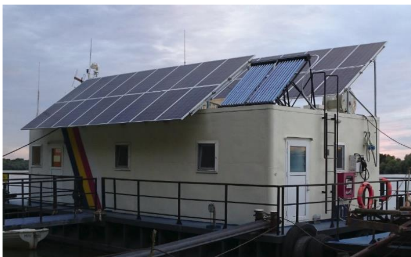
Fig. 1 - Solar installation located on a mooring pontoon in the Danube Delta
